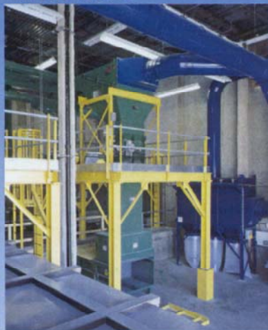
Multiple AIRSCREEN systems with CLEANAIR filtration feeding compactors at a print to mail and shredding facility.
