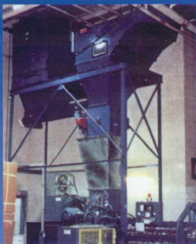
AIRSCREEN System with dust from the CLEANAIR dust collector being directed into the baler chute.
